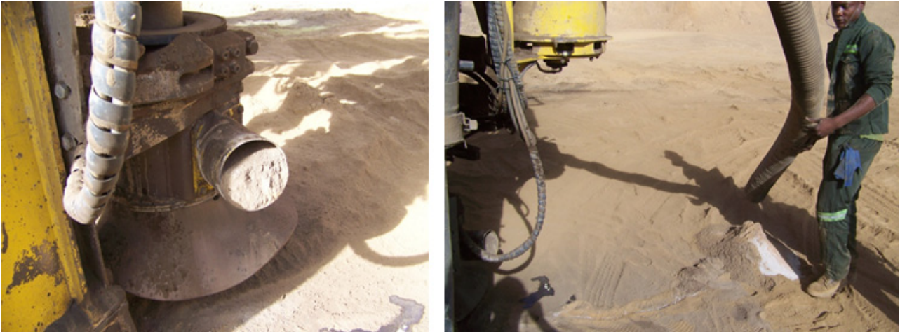
Fig. 7 Blocked dust collector pipe between shroud and cyclone.
