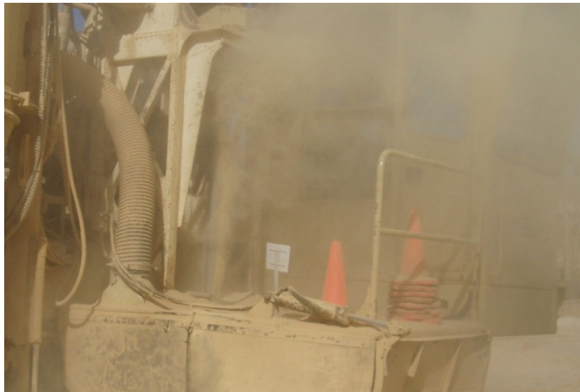
Fig. 5 Dust escaping the sealing ring where the drill stem enters the drill deck.
