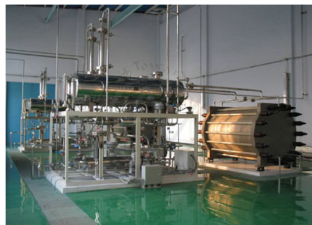
Fig. 8 Hydrogen generation plant.
