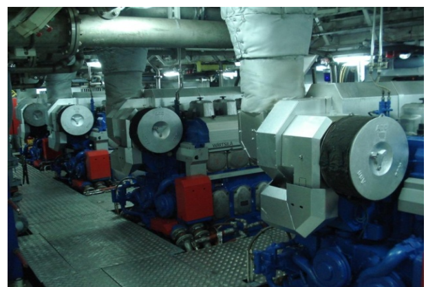
Fig. 4 Diesel generator for power generation.
