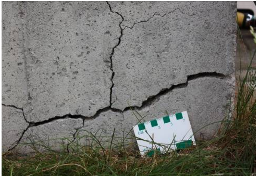
Fig. 1 Cracking in house concrete foundation.
